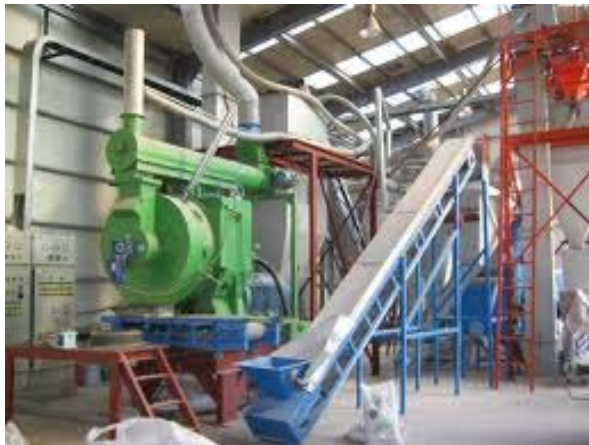
Typical small scale plant
